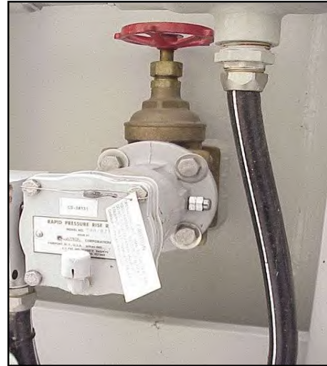
Figure 32 – Photograph of a Sudden Pressure Relay.
