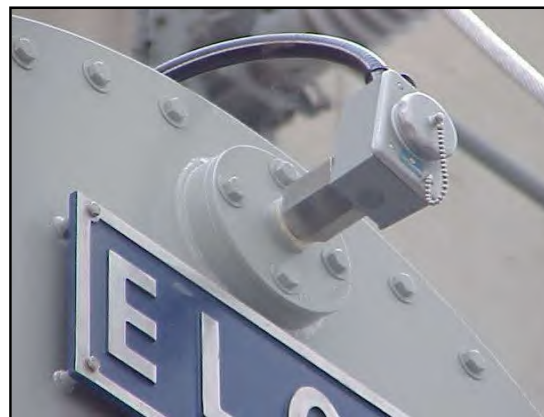
Figure 41 – Photograph of a Bladder Failure Relay.
